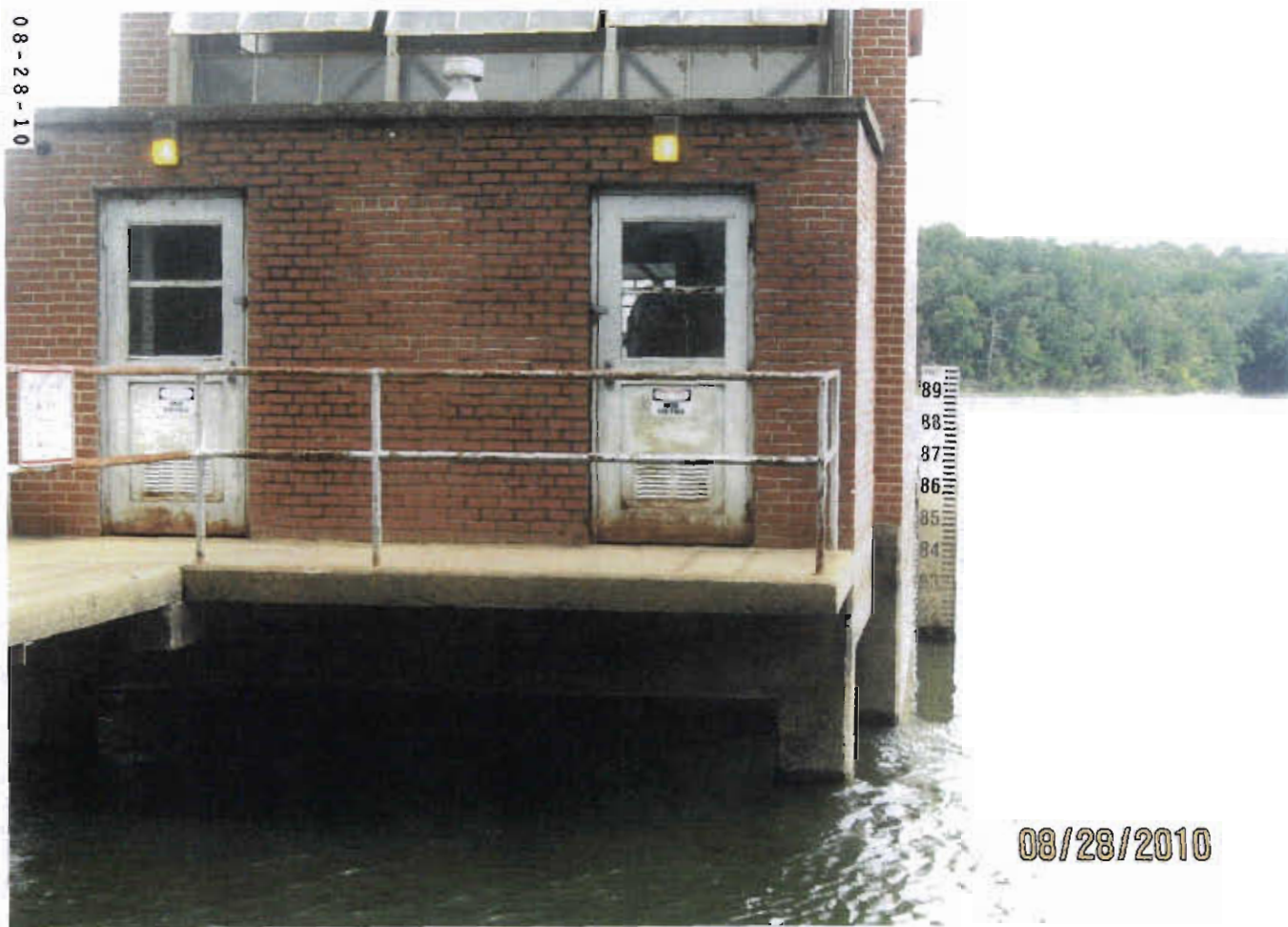
Site #47: Raw Water Intake (Lake Ogletree)
