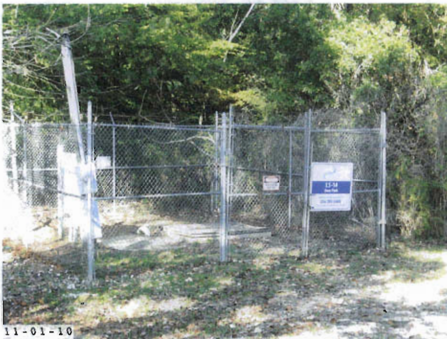
Sites #22 & 23: Lift Stations
